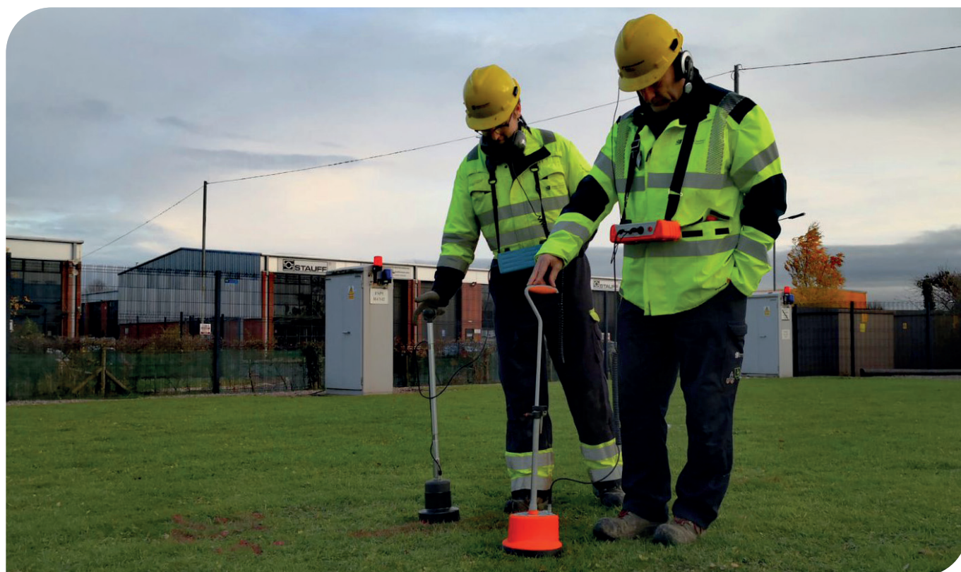
Underground Fault Location Technologies (NIA_SSEN_0037)
